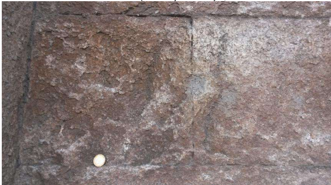
PLATE 8 Detail of Stone Decay on Granite Stone, north facade
