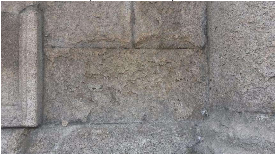
PLATE 10 Detail of Stone Decay on Granite Stone, north façade
