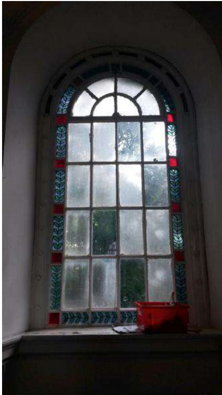
PLATE 46 Typical Upper Level Window to Main Church. Note fogged planes
