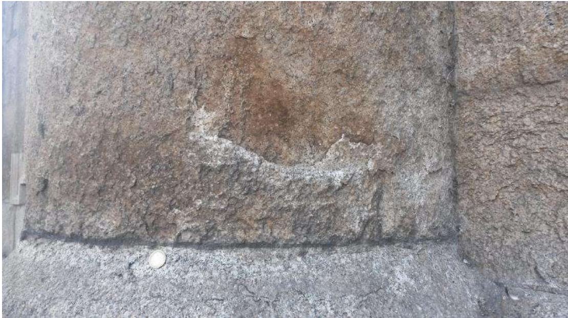
PLATE 9 Detail of Stone Decay on Granite Stone, north façade
