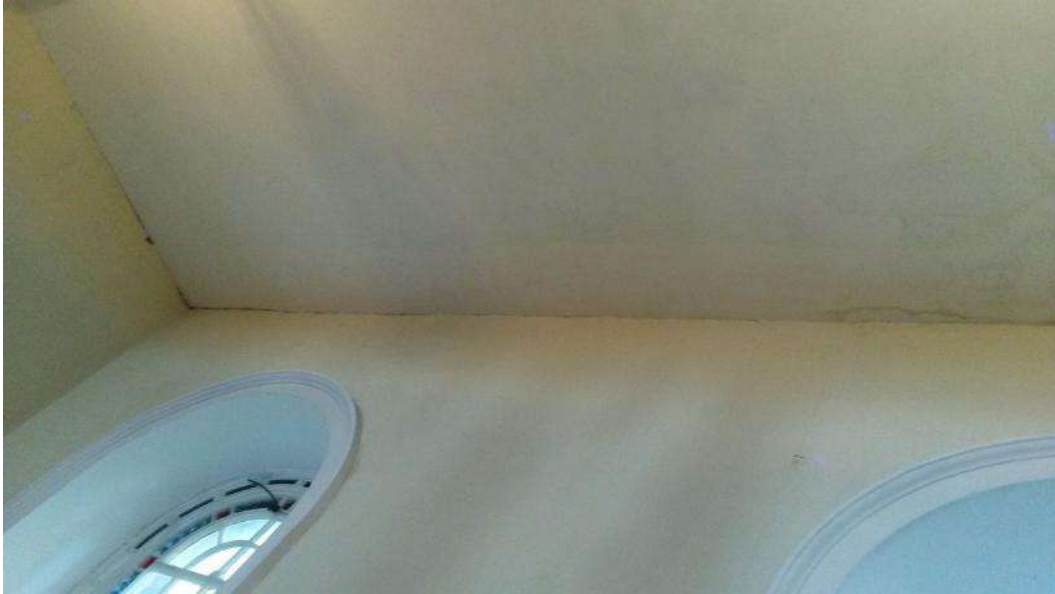
PLATE 40 Damp staining at wall and ceiling junction along southern external wall
