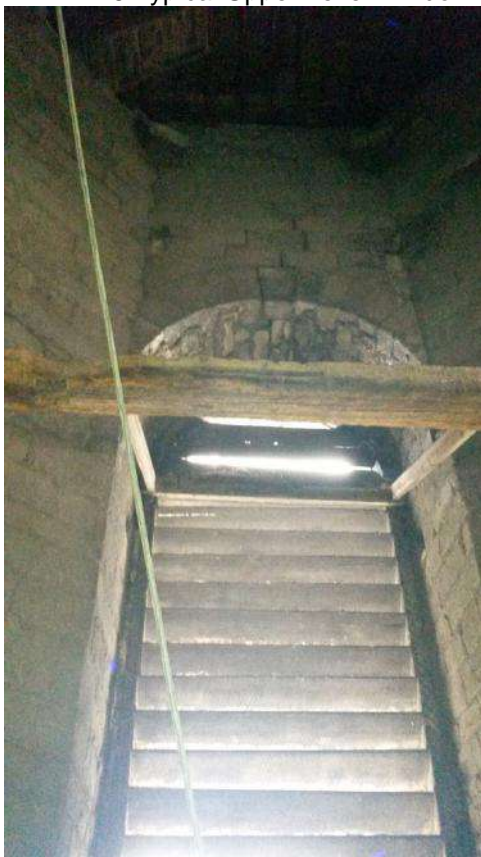
PLATE 47 Slipped Keystone to Arched ope in Belltower
