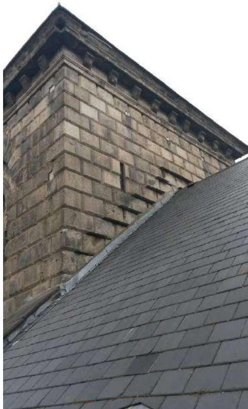
PLATE 22 Projecting slate weatering detail resulting in damage to stone
