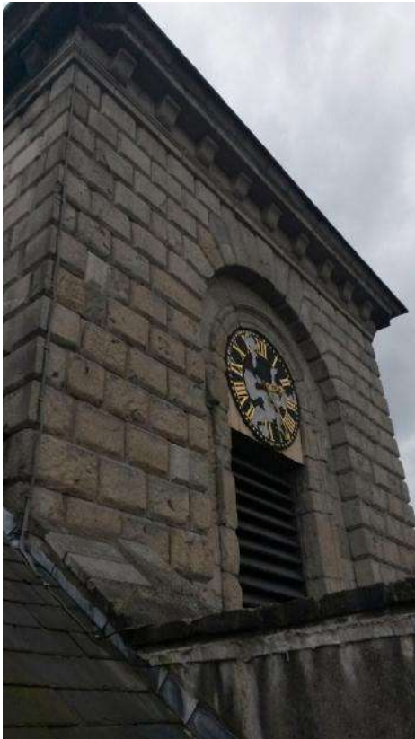
PLATE 23 Belltower, north façade. Clock face on plywood in need of refurbishment,
