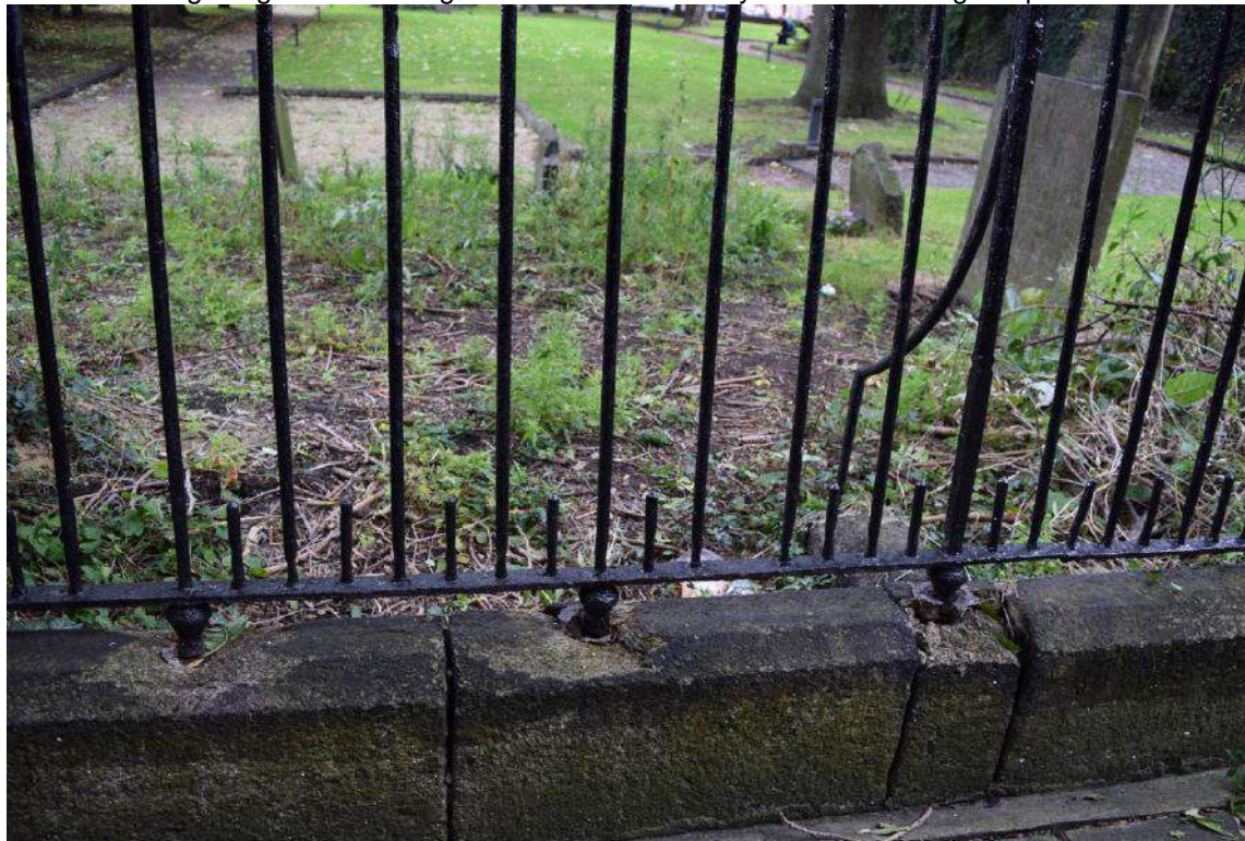
PLATE 26 Southern boundary; expansion of iron filing points have broken granite plinth
