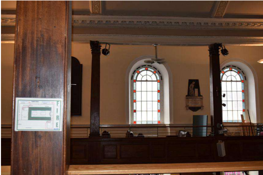
PLATE 42 Bowing of beams between coulms require monitoring
