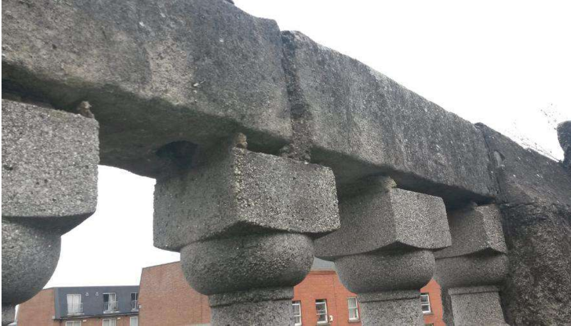
PLATE 30 Mortar fixings for top rail broken away
