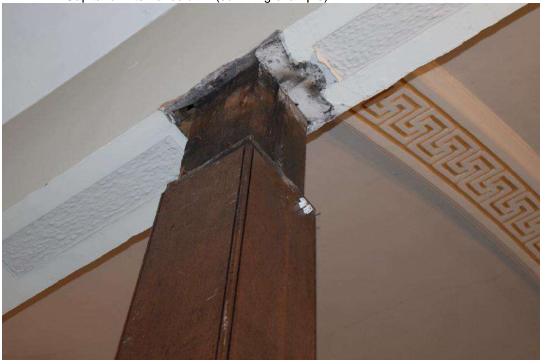
PLATE 45 Damaged/ missing capital of internal column
