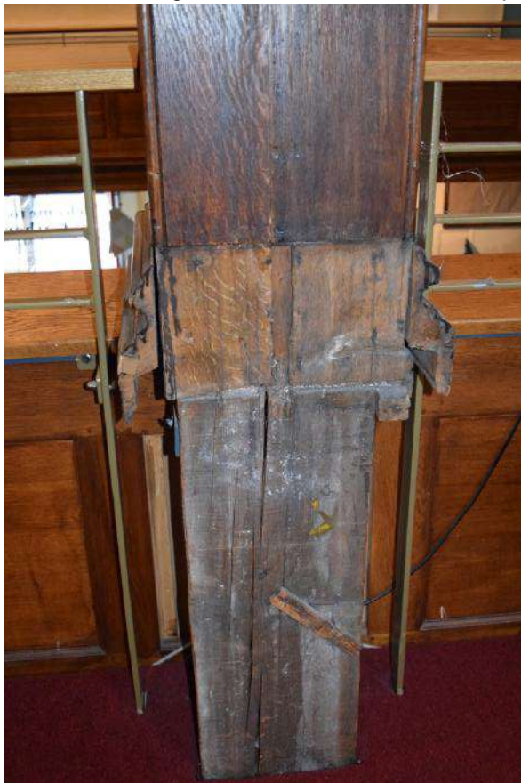
PLATE 43 Damaged timber lining to Timber columns
