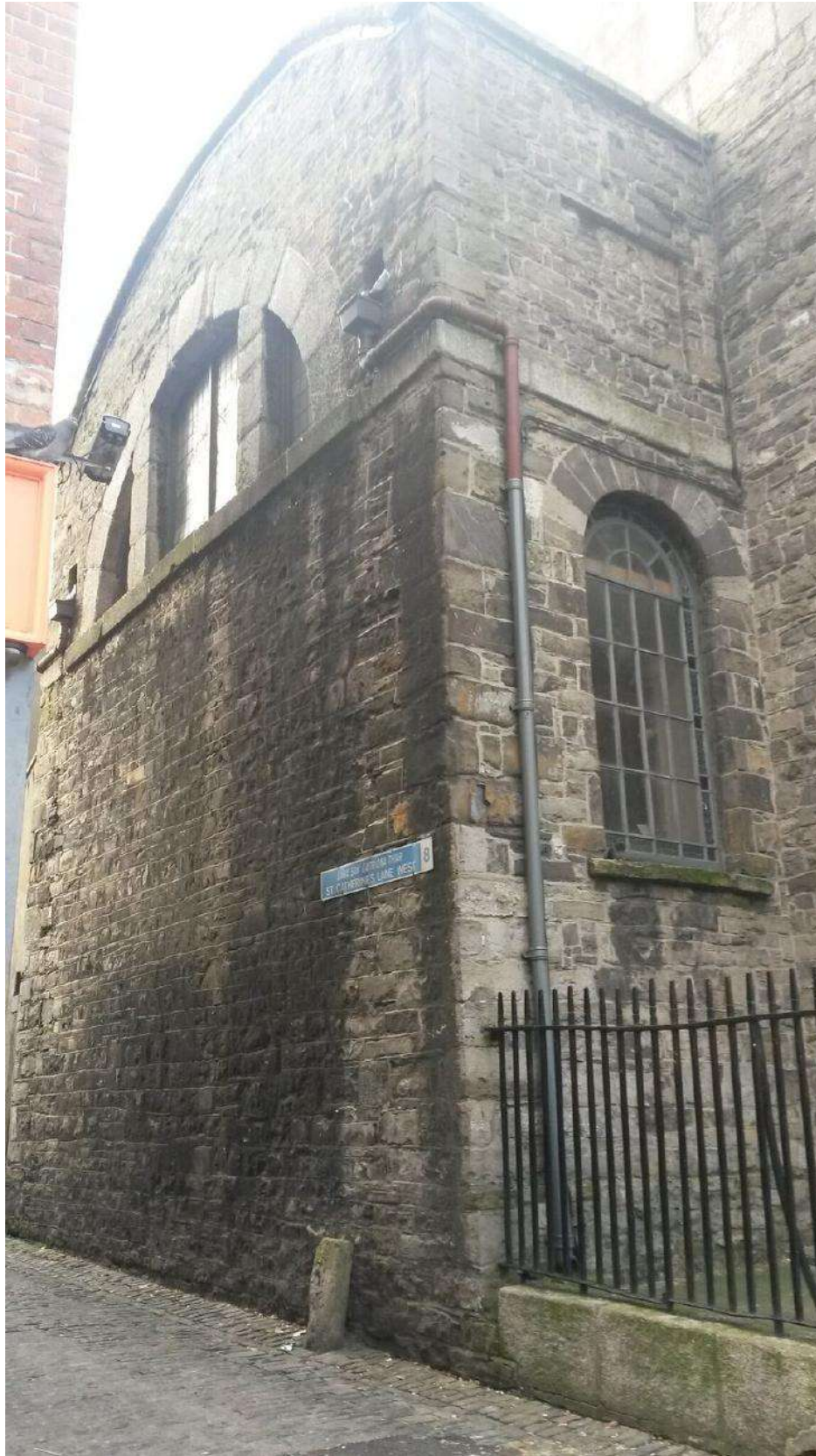
PLATE 18 East Elevation (Note heavy soiling)
