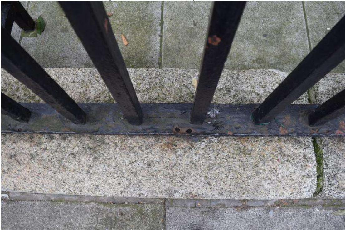
PLATE 24 Coorosion on horizontal bottom rail of iron railings
