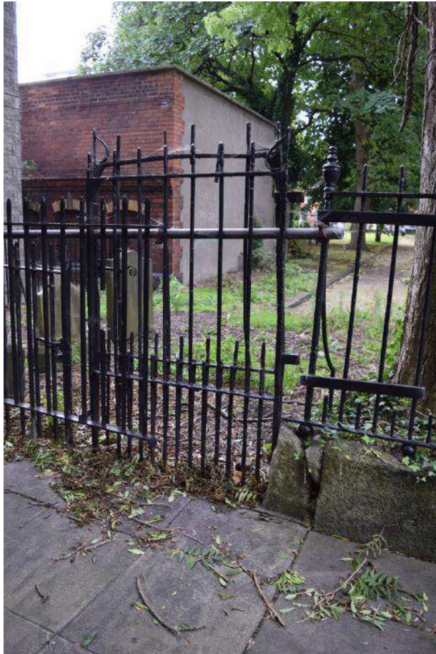
PLATE 25 Original gate and railings to southern boundary with tree damage to plinth
