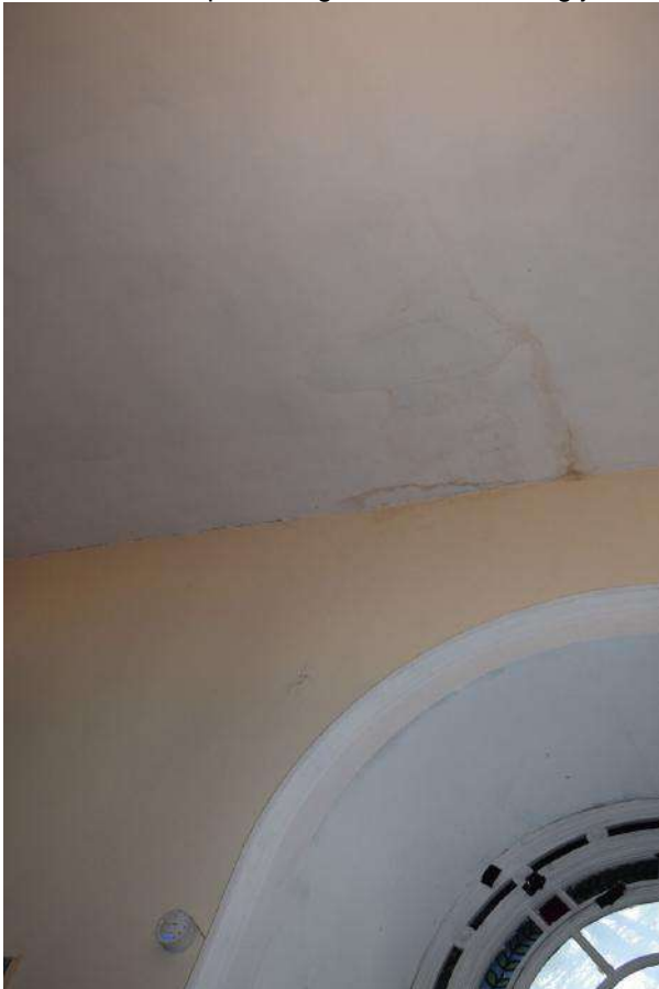
PLATE 41 Damp staining at wall and ceiling junction along southern external wall
