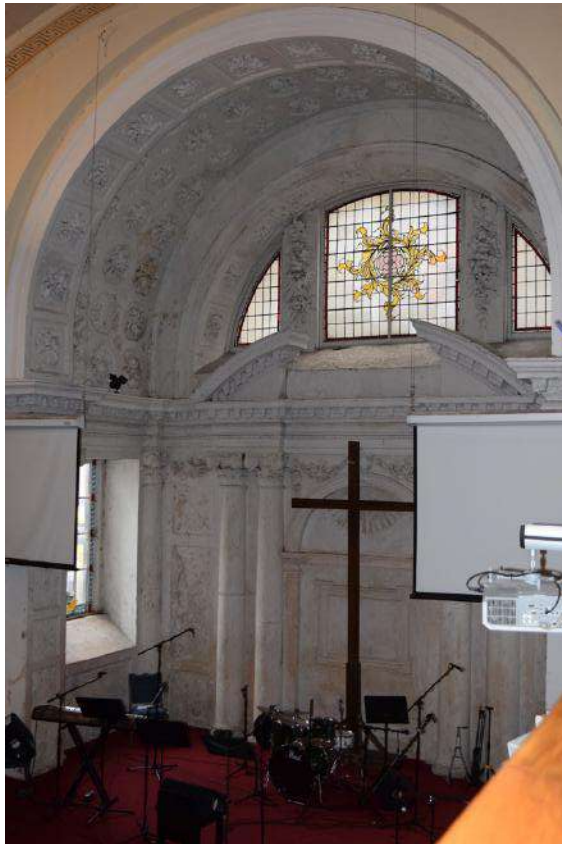
PLATE 35 Chancel – Note cracking to LHS detailed in Fahu Fitzpatrick structural report
