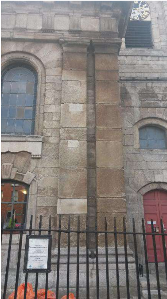
PLATE 7 Severe discolouration to to top RHS façade on Bay 5, North elevation
