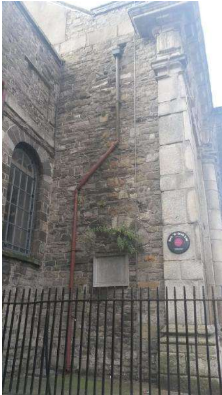
PLATE 19 East façade – Note staining from RWP and vegetation to be remove
