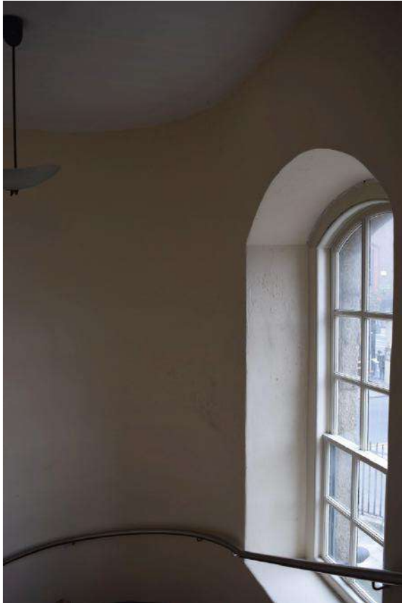
PLATE 39 Damp on wall at landing of stairs
