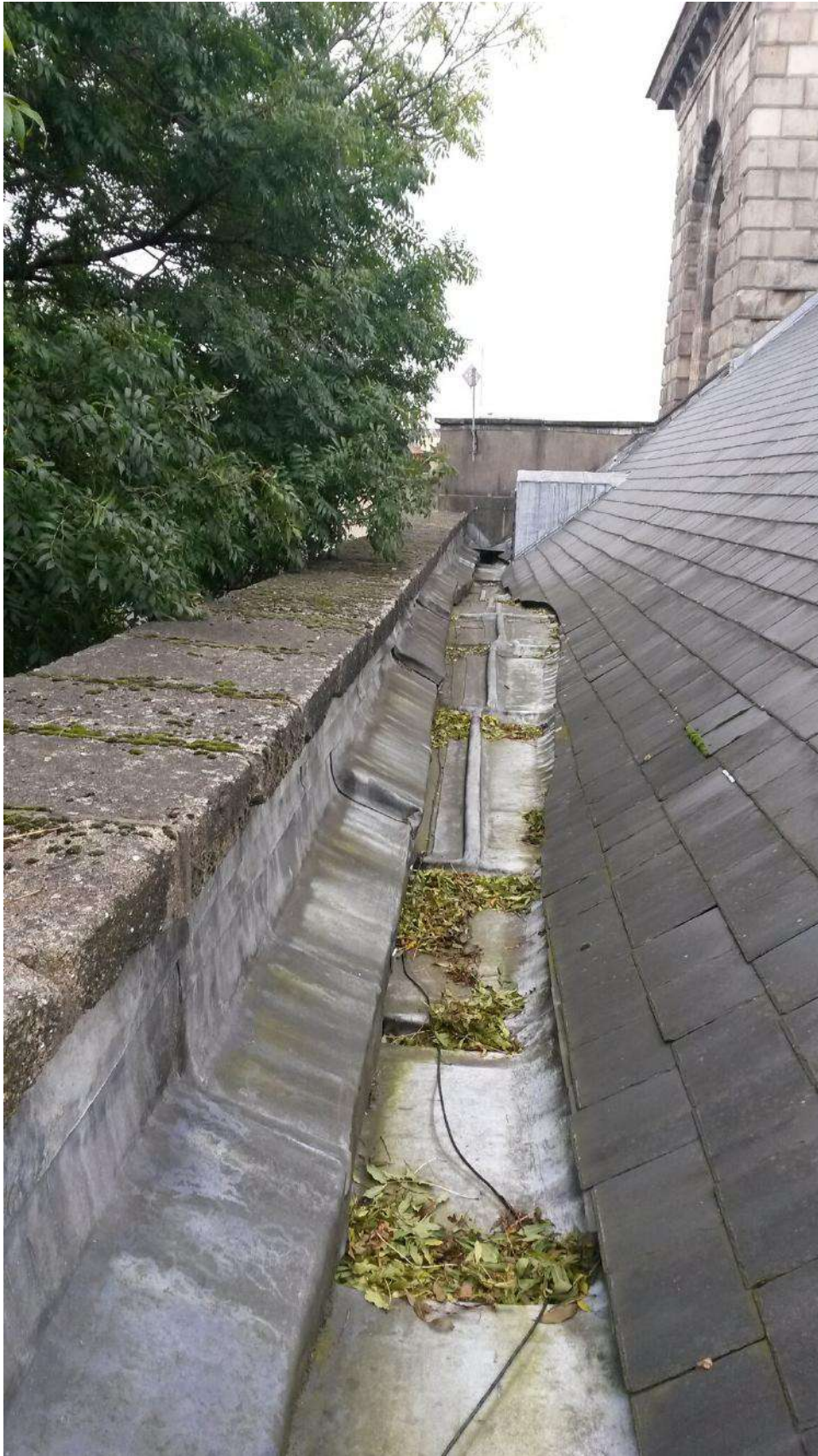
PLATE 33 Overhanging foliage contributing to blocked gutters
