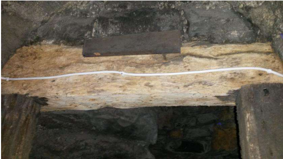
PLATE 48 Beetle infestation to timber lintel in Belltower
