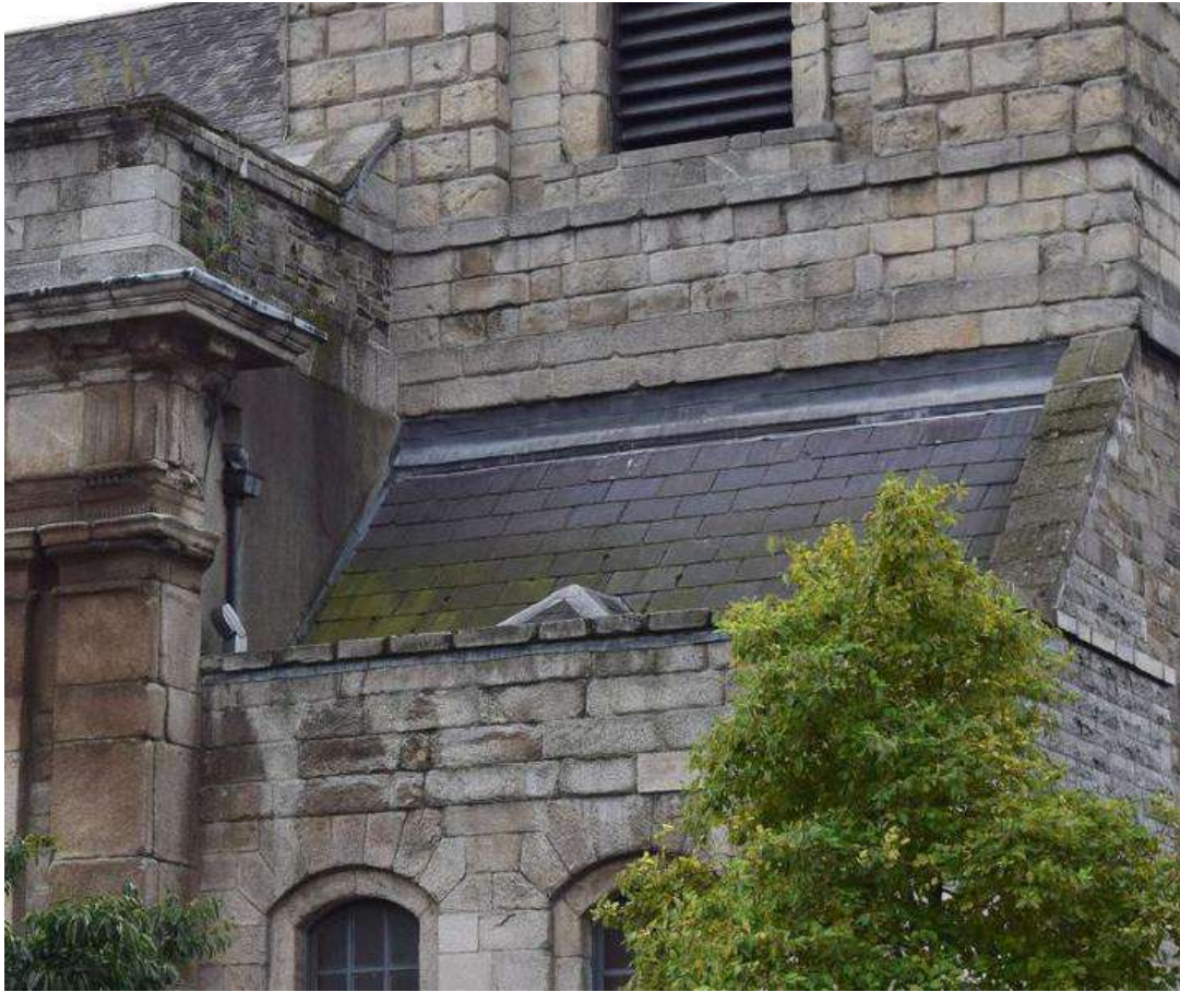
PLATE 32 Moss to be removed from lower roof and gutter checked for leaks/ blockages
