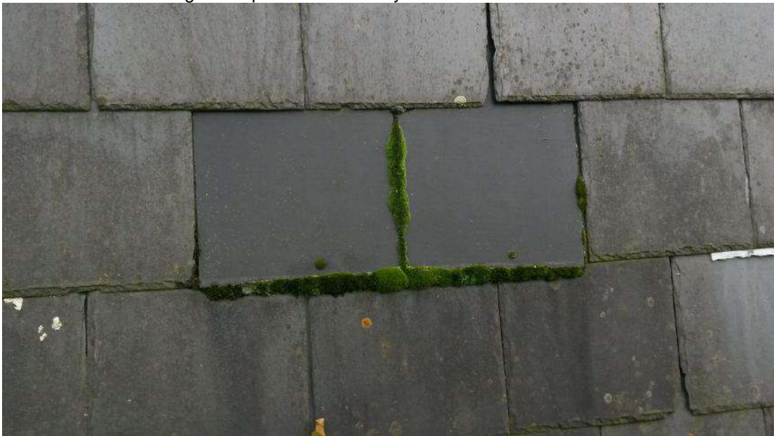
PLATE 31 Remove Moss around roof repair (south facing roof) and inspect for water ingress
